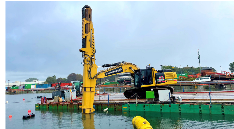
FIGURE 3 Backhoe dredge operating off a pontoon on a German canal construction project.
