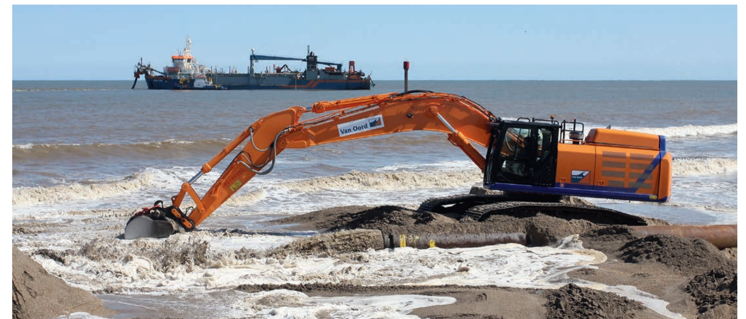
FIGURE 4 Lincshire Beach Nourishment scheme being undertaken by Van Oord. Photo @ Van Oord.
