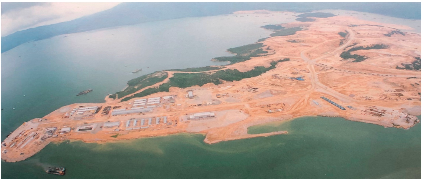
FIGURE 2 Aerial overview of the two islands merged into one to create Chek Lap Kok airport.
