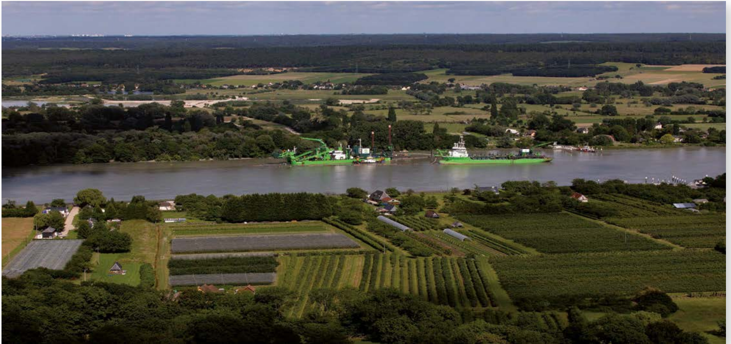
The dredgers Reynaert and Amazone performing deepening works on the River Seine.
