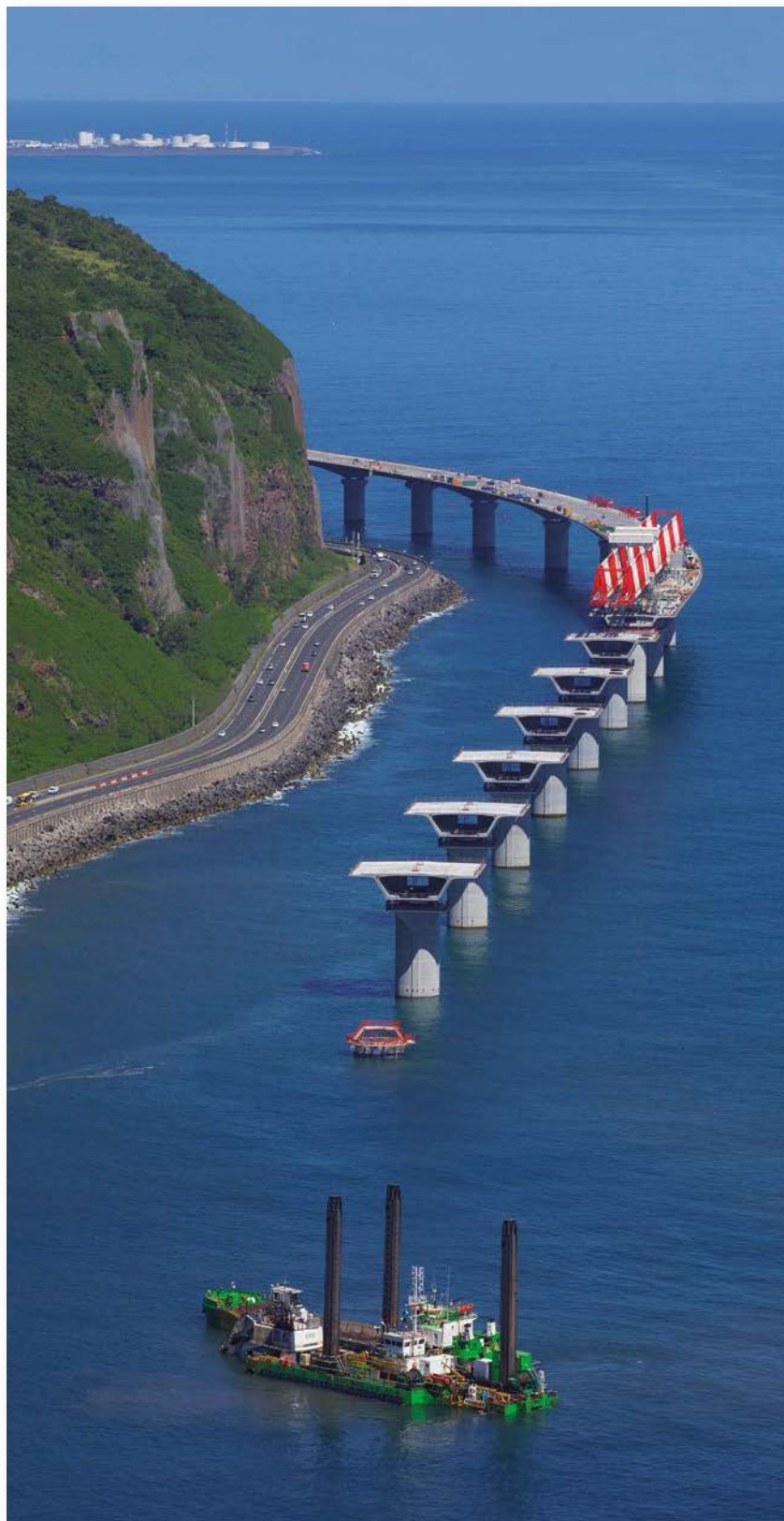
The new coastal road being built at Reunion Island. Read more about this project in Terra et Aqua #151, page 27.
