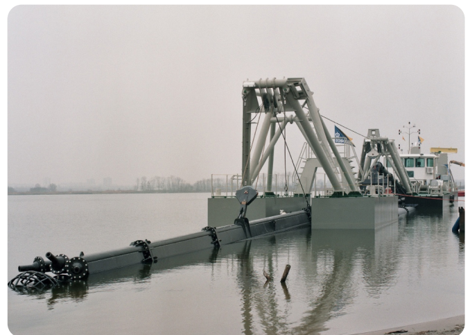
This Plain Suction Dredger (PSD) from Boskalis is a hydraulic dredger using hydraulic centrifugal pumps to provide the excavating force.
