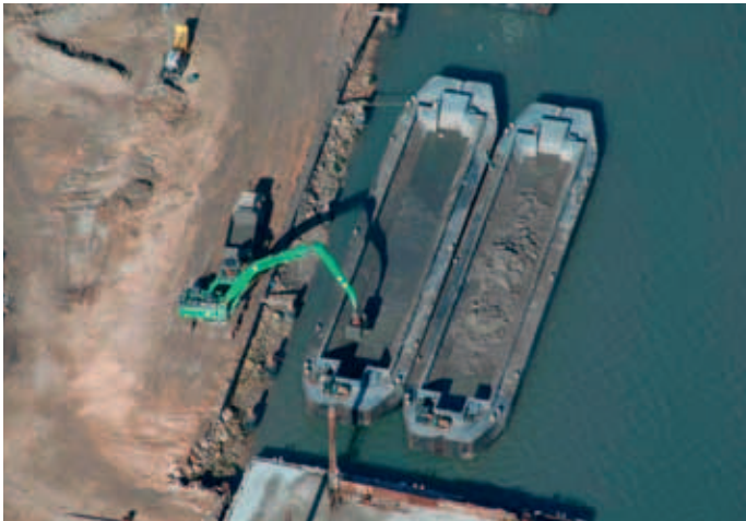
TOP. Floating pipelines are used to transport dredged sand to the placement site.
