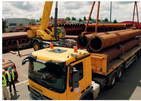
Figure 9. In the new procedure, pipes are lifted by C-hooks which are attached to soft slings.
