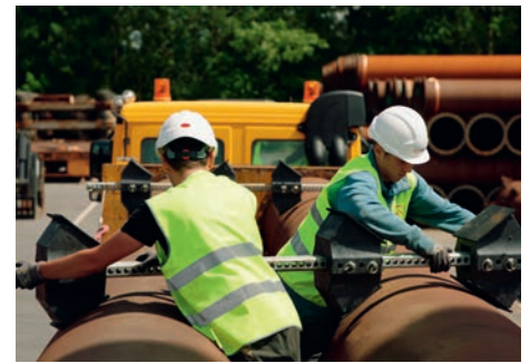
Figure 4. Workers place a mid-section cradle atop the first layer of pipes which will support the second tier of pipes.
