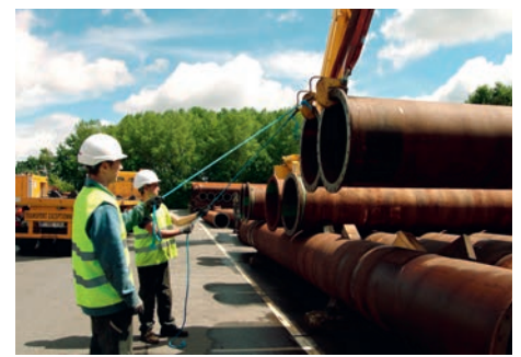
Figure 7. With a guideline in hand, riggers manoeuvre pipes into position. To hook off, riggers simply pull on the guideline after the pipe is in place.
