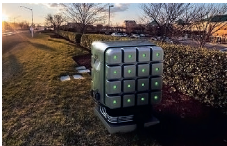
Figure 6. The Power Cube from Redox Power is a SOFC fuel cell being used as a UPS system.
