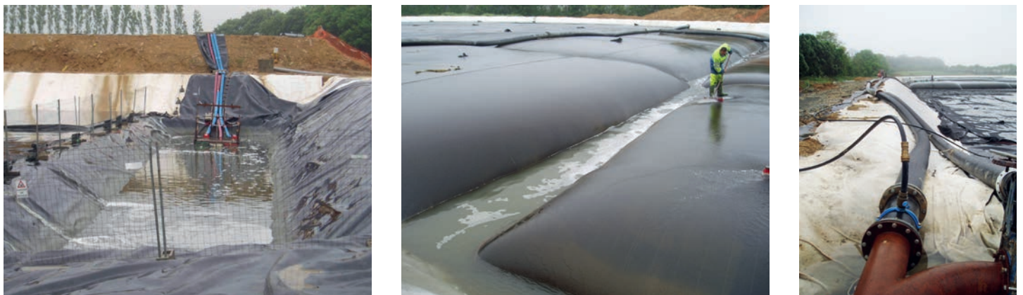
Figure 8. Water exited the dewatering tubes and flowed by gravity to the low point, and was then pumped to a retention area where turbidity was continuously monitored.
