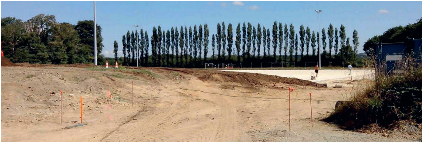
Figure 9. During construction, the soccer stadium (white area) can be seen from the entry of the parking area.
