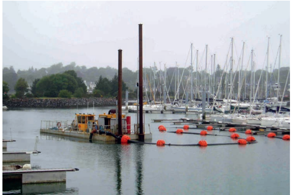
Figure 5. A dredger pumps the sediment at Port-La-Fôret harbour into a floating pipeline.
