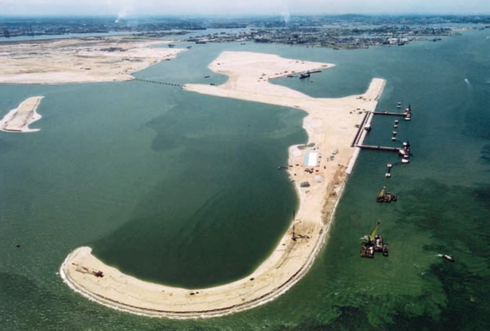
Figure 1. Work on Jurong Island (Phase 4) Reclamation. Seven existing islands were linked up to create one large island, which increased the land area of Singapore by 540 ha.
