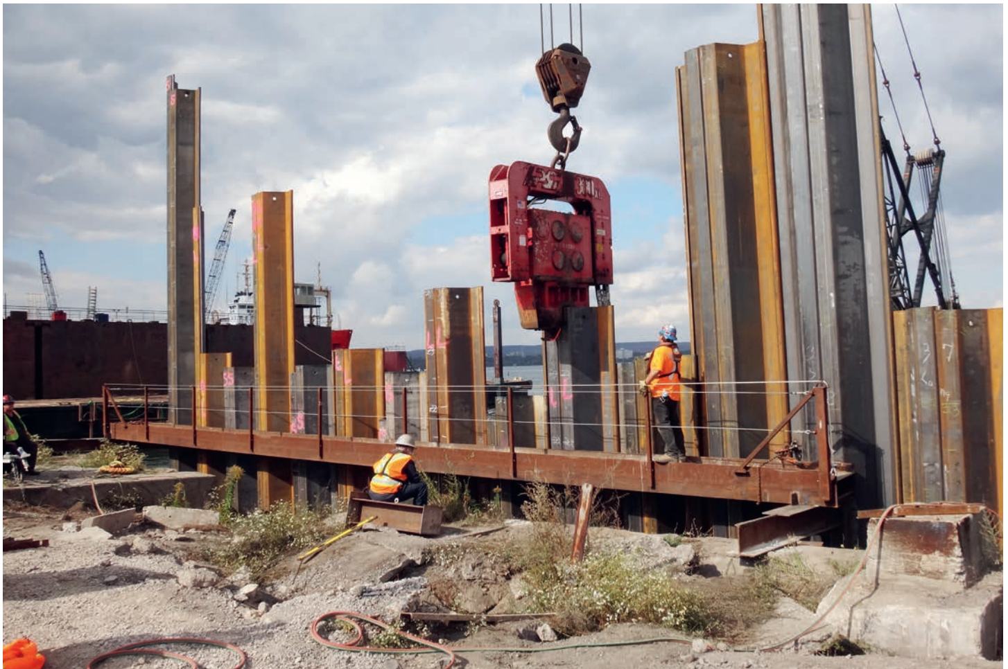
Figure 1. Installation of the face wall sheet pile at Pier 15 East (Heddle Marine) on 7 October 2015. Photo Riggs Engineering Ltd.
