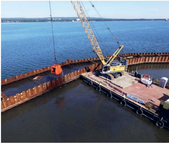
Figure 3. Mechanical dredging moves contaminated sediment from between the double walls of the ECF into the ECF containment cell. Photo McNally Construction Inc.
