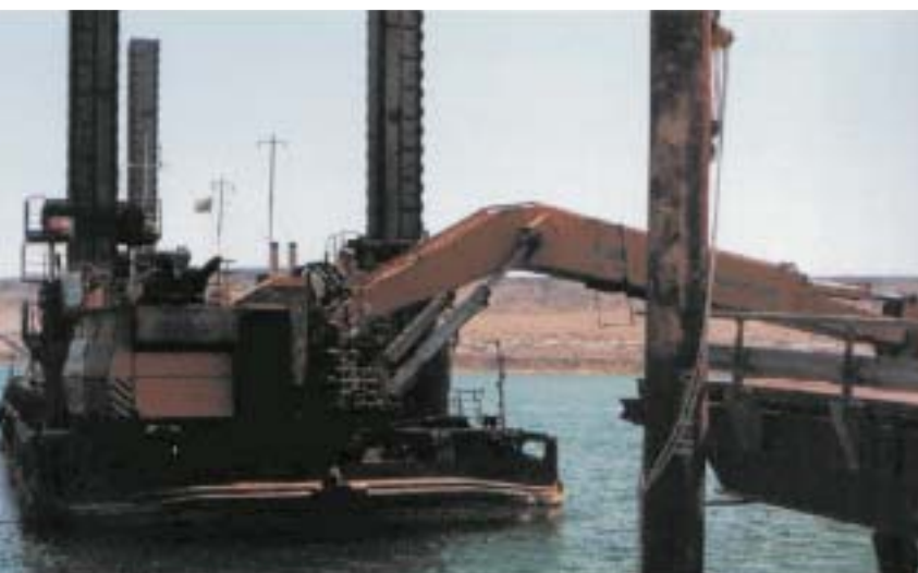
Figure 10. Meeting standards and goals during the first year was made more difficult because of the old and ill-maintained "local" equipment – barges, tugboats and a jack-up platform equipped with a hydraulic excavator – rented from Russian suppliers.
