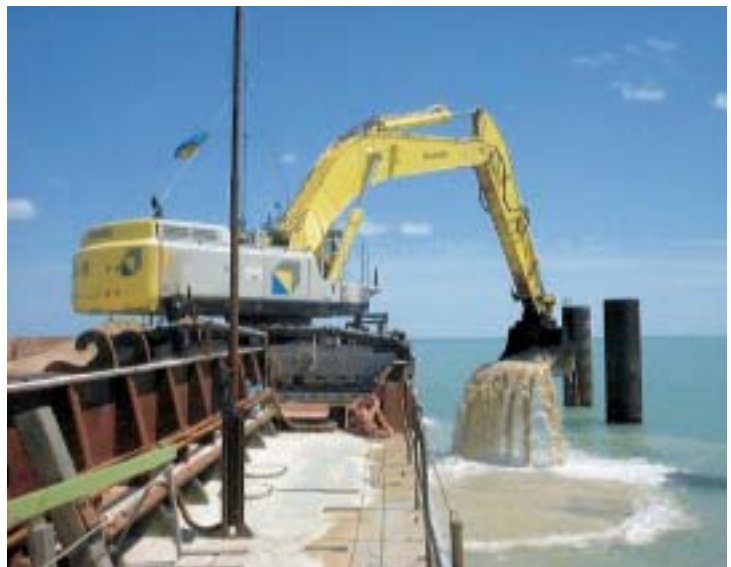
Figure 12. A hydraulic excavator is equipped with its own on-board satellite positioning equipment and Crane Monitoring System (CMS) to assist the operator in the underwater construction activities.
