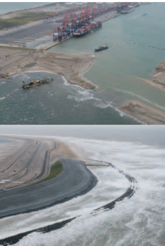
Figure 29. Top: CSDs Edax and Zeeland II at work while creating the passage to Maasvlakte 2 from the Yangtzehaven. Below: Stormy weather conditions at the stony dune and block dam, November 25, 2012.
