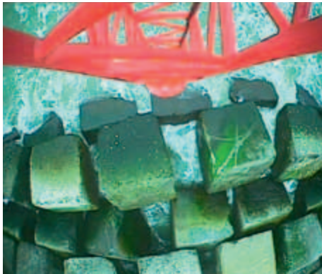
Figure 17. Image from the frame-mounted camera.
