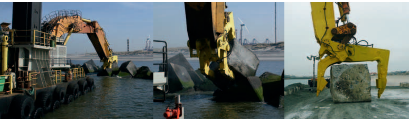
Figure 24. Left: Backhoe Wodan extracting a block from the Maasvlakte 1 block dam. Middle: Close up of the Wodan’s ripper tool holding firmly to a 40-tonne concrete block. Right: A 40-tonne block is safely released on to the transport barge.
