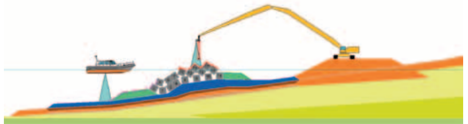
Figure 20. Laser scan survey of the crest blocks. Additionally the survey vessel will survey the remaining part of the 1-10 tonne toe structure.
