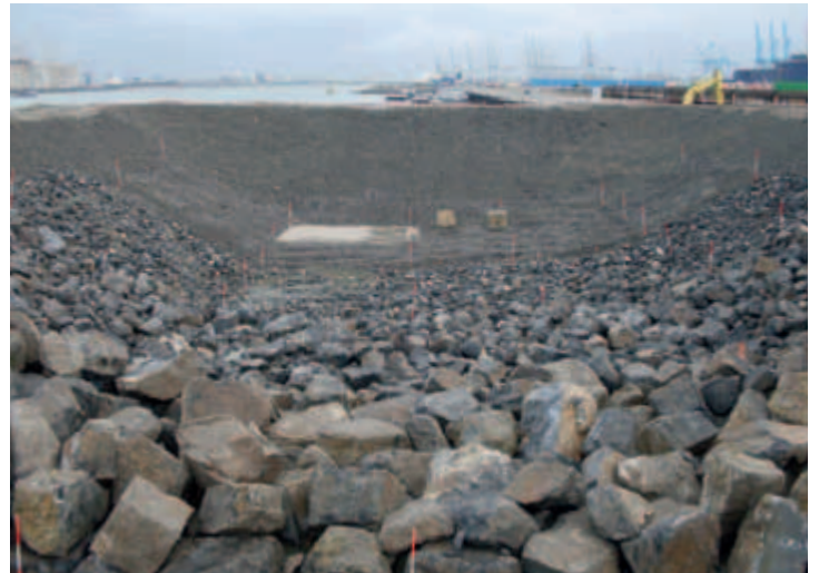
Figure 4. Test pit after dry sand excavation and filled with rock grades that will be used during construction of the hard sea wall. The flat sand area with concrete plates was used for calibration purposes.
