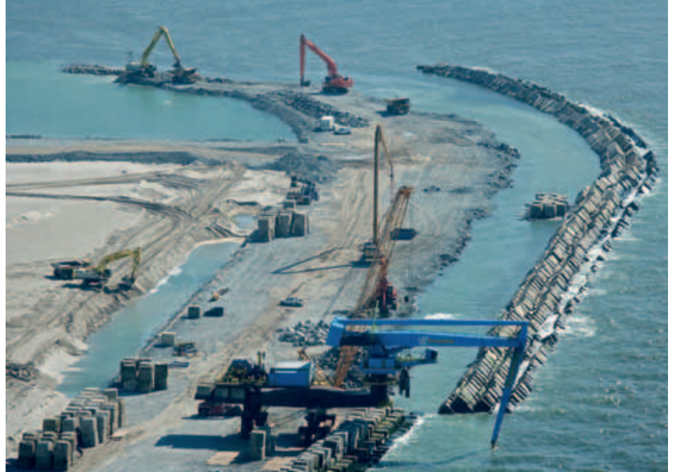
Figure 10. The Blockbuster standing behind the temporary protection of the work road and placing a 40-tonne concrete block in the hard seawall.
