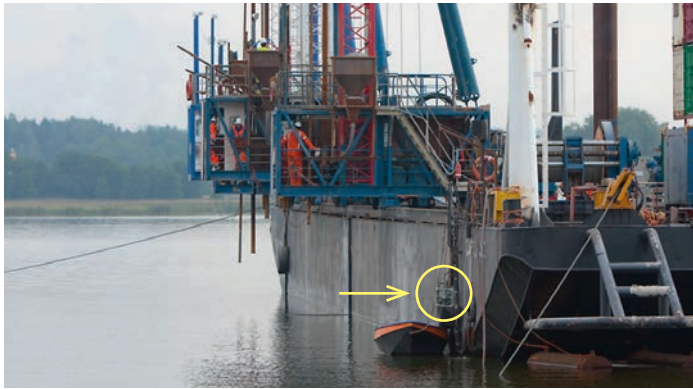
Figure 6. FaunaGuard in Norrköping (Sweden) hanging off the drilling and blasting barge before deployment.
