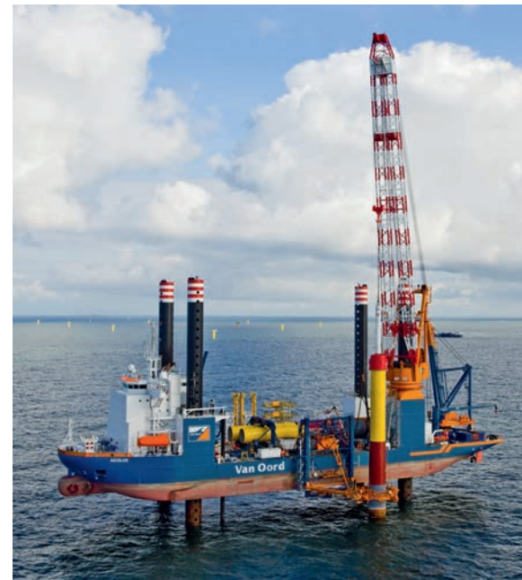
Figure 8. Installation vessel Aeolus at work during the construction phase of the Eneco Luchterduinen Wind Farm in the Dutch North Sea.
