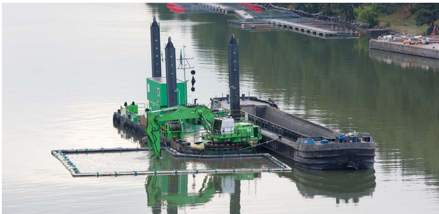
Figure 3. The dredger, Ijburg , in combination with a level-cut clamshell bucket was utilised to perform the dredging works in the Valdemarsviken fjord.
