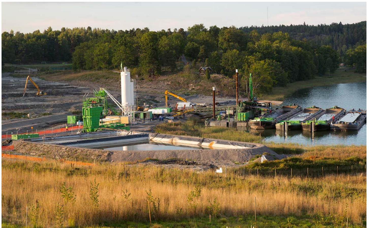
Figure 8. From right to left: Barges are unloaded; the mixing plant; and the stabilised sediments are spread into the backfilling area. At the front of the image, the water buffers from supernatant and run-off water can be seen.
