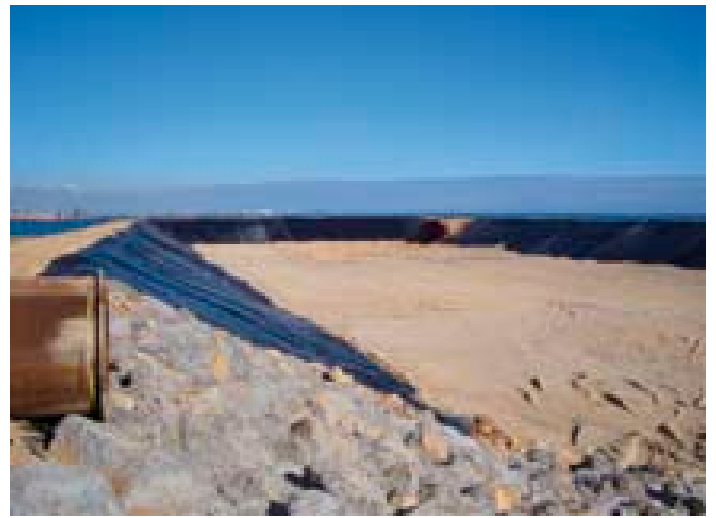
Figure 7. View of the main settlement pond.
