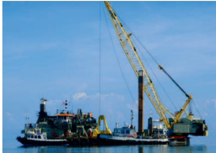
Figure 3. Work in progress at the Falmouth Cruise Terminal. Grab Dredger Packman was responsible for removing the soft dredged material during the first phase.
