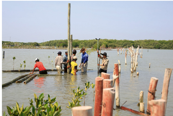
Figure 3. Construction of permeable dams by local contractor under supervision of the BwN team. Training-on-the-job is an important part of the BwN approach. (Photo: Tom Wilms)
